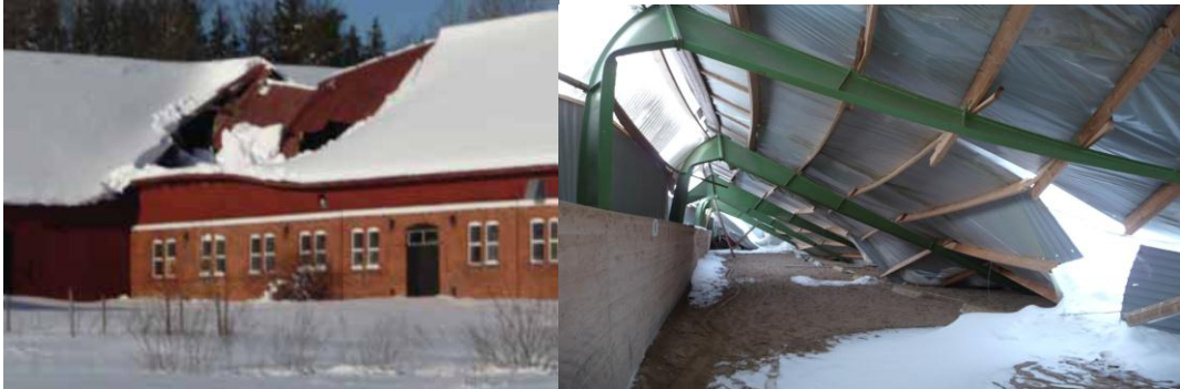
FIGURE 3. Left: Roof collapse caused by high snow load in the roof valley. Right: Collapsed roof of a riding arena due to undersized 3-hinge frame structure. The frame was dimensioned for too low snow load (wrong snow zone).
