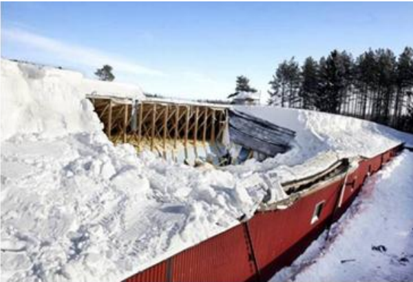
FIGURE 2. Unsymmetrical roof snow load due to prevailing wind from the left side in the picture when snowing, resulting in collapse.
