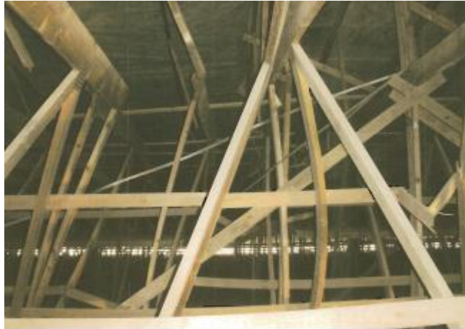
FIGURE 5. Insufficient braced compressed diagonals of W-trusses. Progressive collapses of the trusses has also been initiated.
