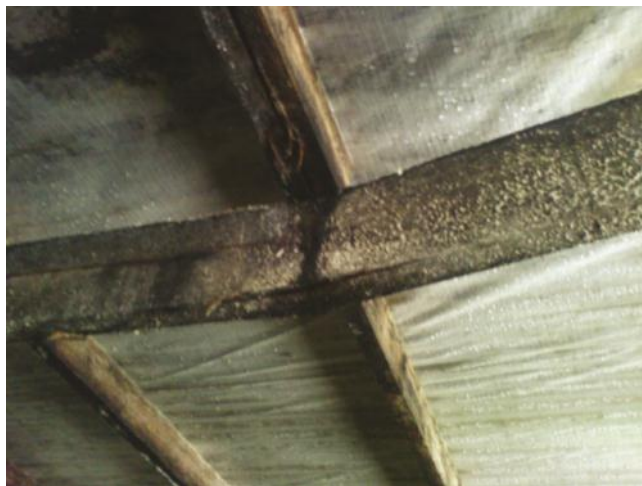
FIGURE 6. Insufficient ventilation of the livestock house has made the roof ridges become rotten resulting in decreased strength. Extreme snow load revealed the bad conditions.
