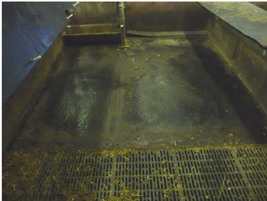
Figure 5. When removing the hard rubber mats after 10 months, a lot of moisture was found beneath. (Photo: R. Westin)
