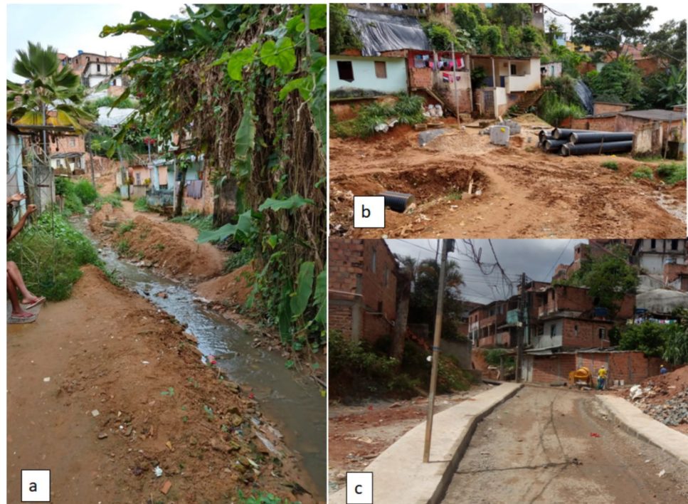
Fig. 1 Infrastructural intervention in Pau da Lima, Salvador-BA, Brazil; a typical open sewer in Pau da Lima, b cross-sectional area of an aspect of the community during the intervention, and c modification of sidewalks to reduce sewer water accumulation
