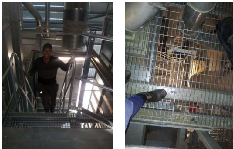
Figur 8. Spannmålsgårdens torksiloanläggning. The new dryer silo facility at the grain farm.
