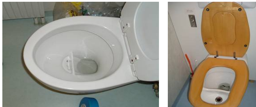
Fig. 2. Double flush urine diverting toilets of different designs, Sweden (photos: C. Niwagaba, 2005).
