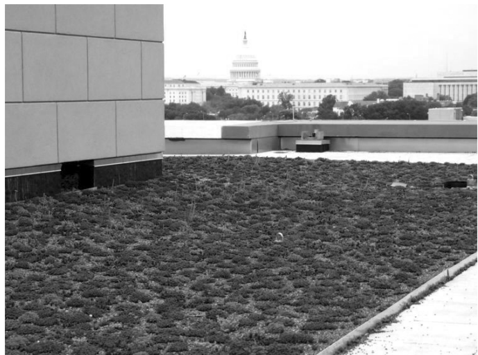
Fig. 1 Greenroof on Department of Transportation, Washington DC, USA (photo by www.greenroofs.com/projects/pview.php?id=280 )
