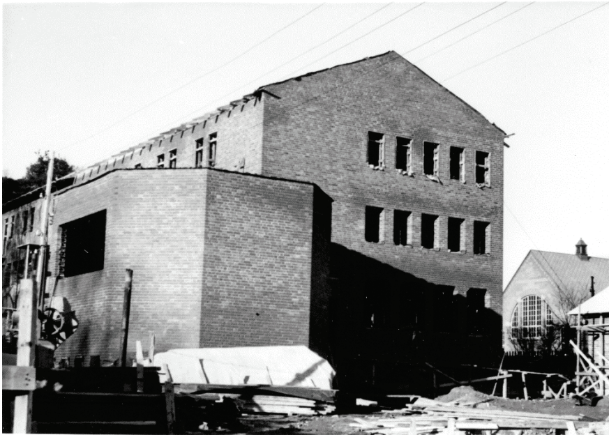
Figure 2. In 1945, Nils Lagerlöf's department moved into a new, purpose-built building on the campus of the Veterinary College. The building, seen here under construction, is also a fitting symbol of Lagerlöf's institution-building ambitions. Photographer unknown. From the Swedish Veterinary Museum's photography collections.
