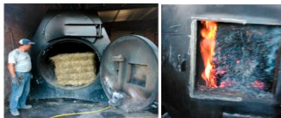
Figure 8. A boiler where a biomass bales are used in Spain [12].
