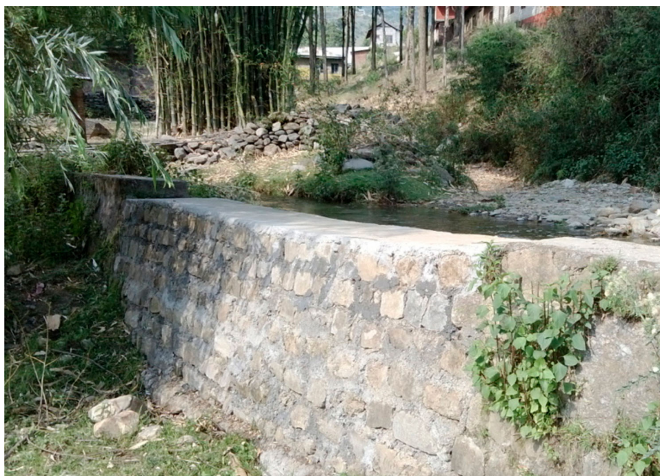
Figure 6. The upper layer of the retaining wall was repaired following damage of a storm, helping to ensure continued water availability downstream.
