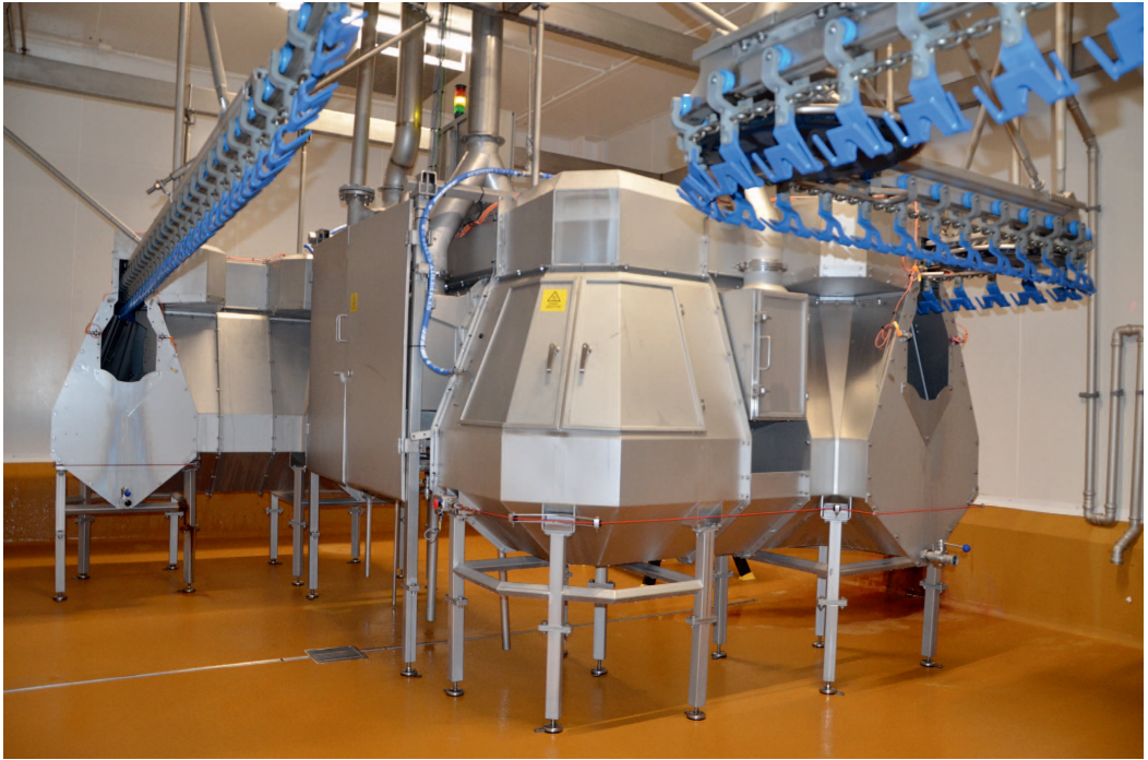
FIGURE 1. Ultrasound-steam chamber installed in the slaughter line of a large-scale broiler chicken processing plant.
