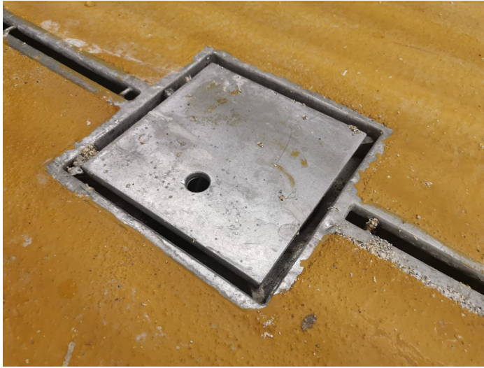
Figure 15. Contaminated drain in a slaughterhouse (photo by author).
