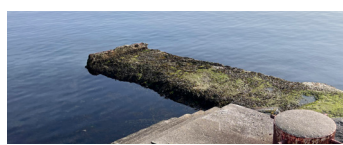
6. Manhole in tidal zone overgrown with algae
