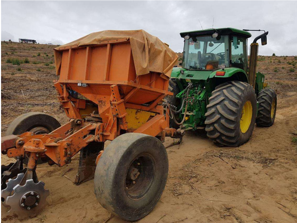
Site preparation equipment pulled by a standard farm tractor. Photo: Mikael Lundbäck
