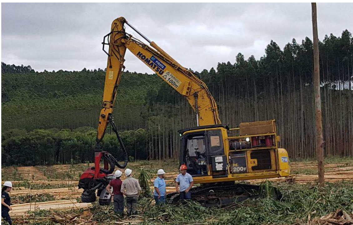
Eucalypt harvest area with several excavators with harvester heads. Photo: Mikael Lundbäck
