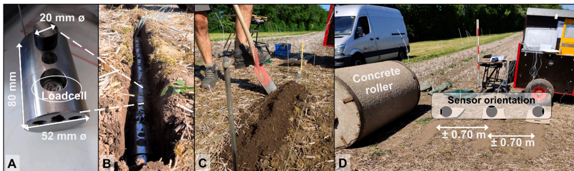
Fig. 3. Overview of installation of the stress sensors. See Sections 2.3 and 2.4 for explanation. Photos A–C by Loraine ten Damme, photo D by Jens Bonderup Kjeldsen.
