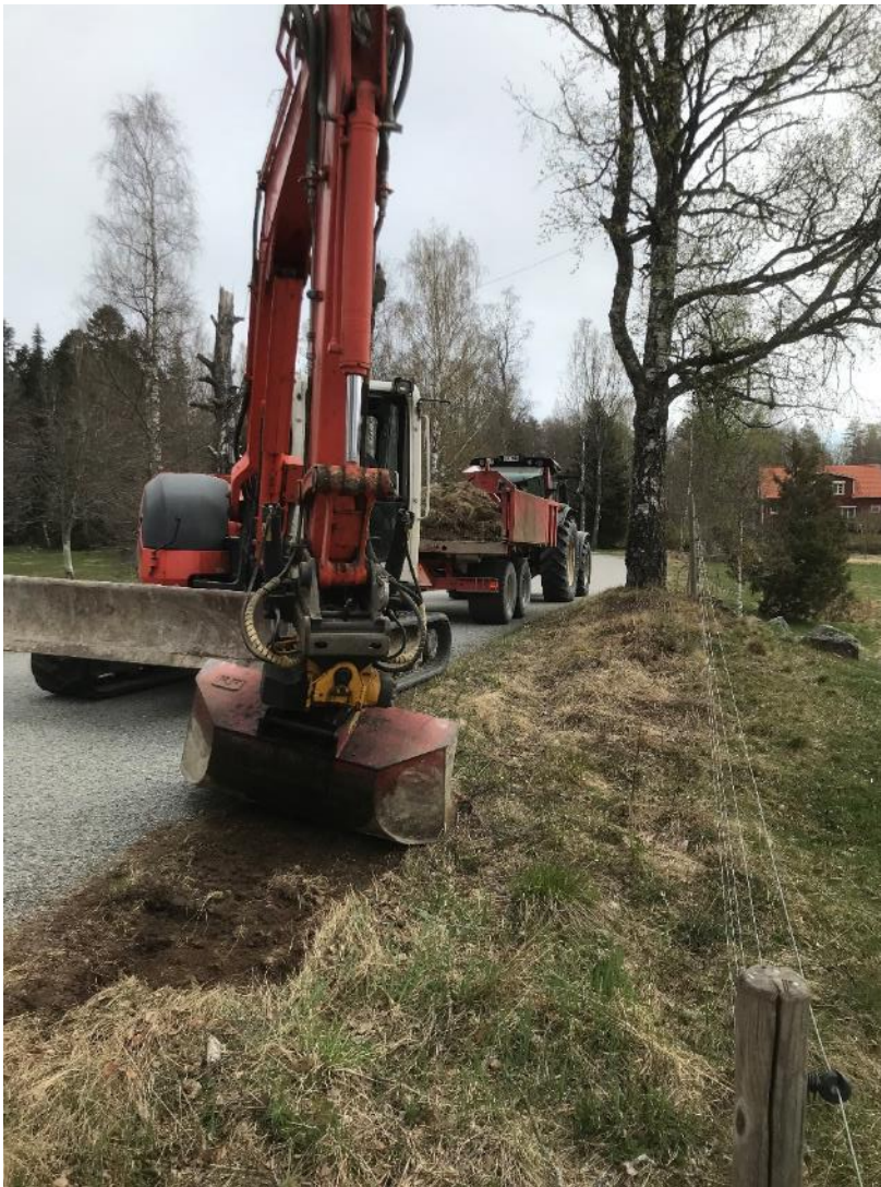
Figure 41. Regular road maintenance include many activities that cause physical disturbance to the ground and field layer. Grönbo, province of Västmanland, Sweden. Photo Jan Olof Helldin.
