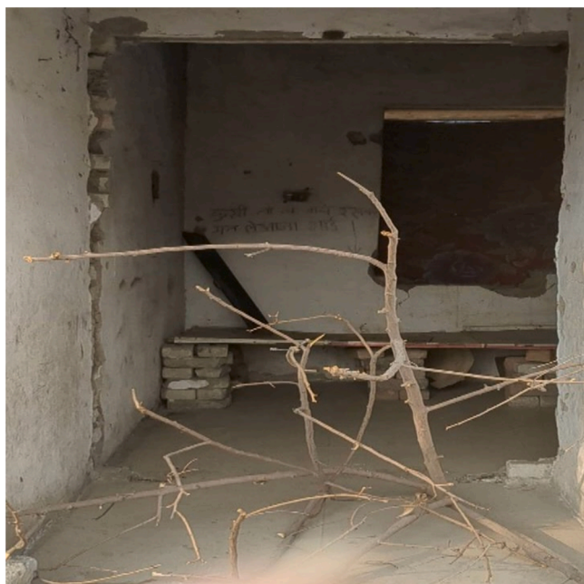
Fig. 2. Picture taken by one of the authors of a security hut at the abandoned Banki Colliery on the outskirts of Korba town on 23 November 2023.
